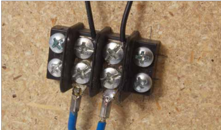
14. Large gauge (16 AWG) stranded bus connected through a barrier terminal strip to a smaller gauge (20 AWG) solid wire.
