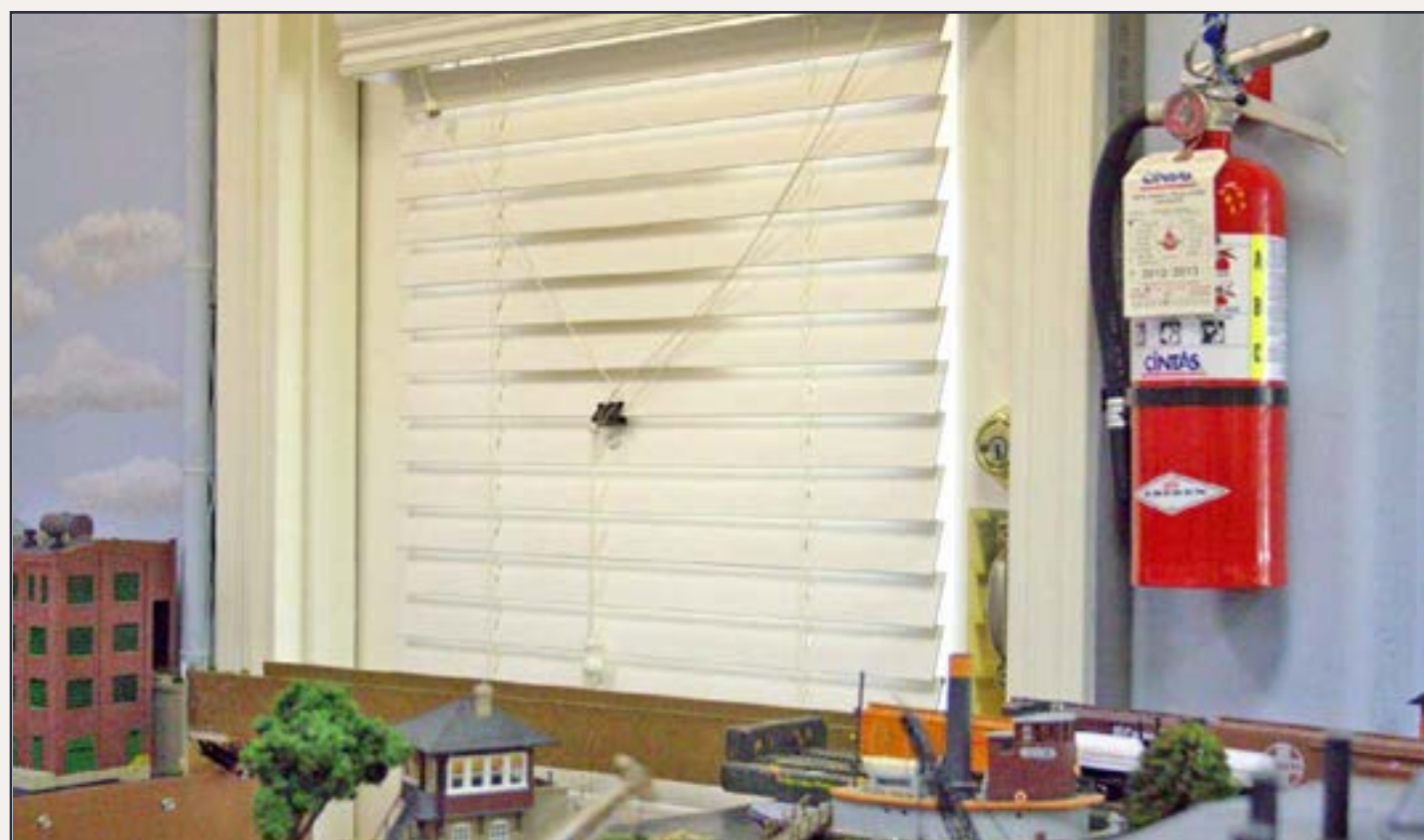
4: Fire extinguisher installed near the door at the Pebble Creek club layout.
