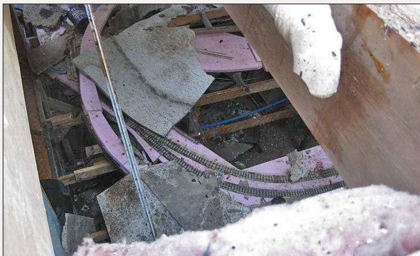
2: After the fire – a view of Peter’s layout from outside the house – photo courtesy of Peter Herron.
